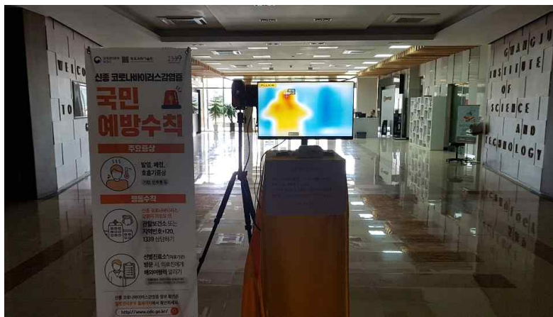
(Photo 2) Installation of a thermal imaging camera in major buildings at GIST
