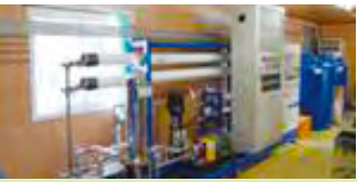
SWRO Pilot Plant
